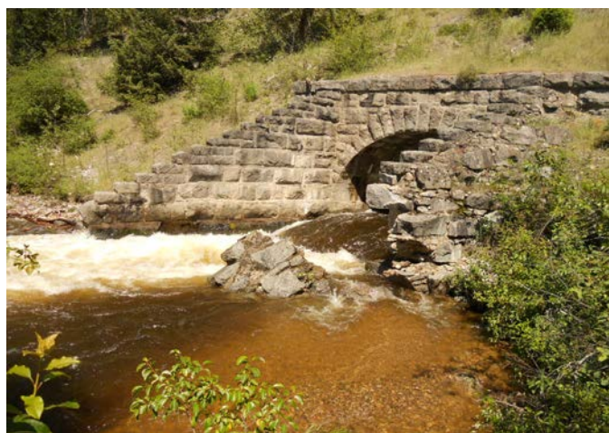
Downstream View, showing failed wingwall
